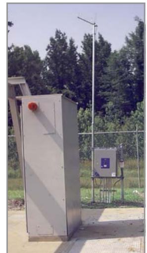
Lift Station Control with DFA Remote Terminal Unit.
